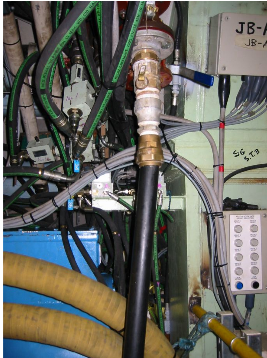
A liquid hose connection point & emergency valve
